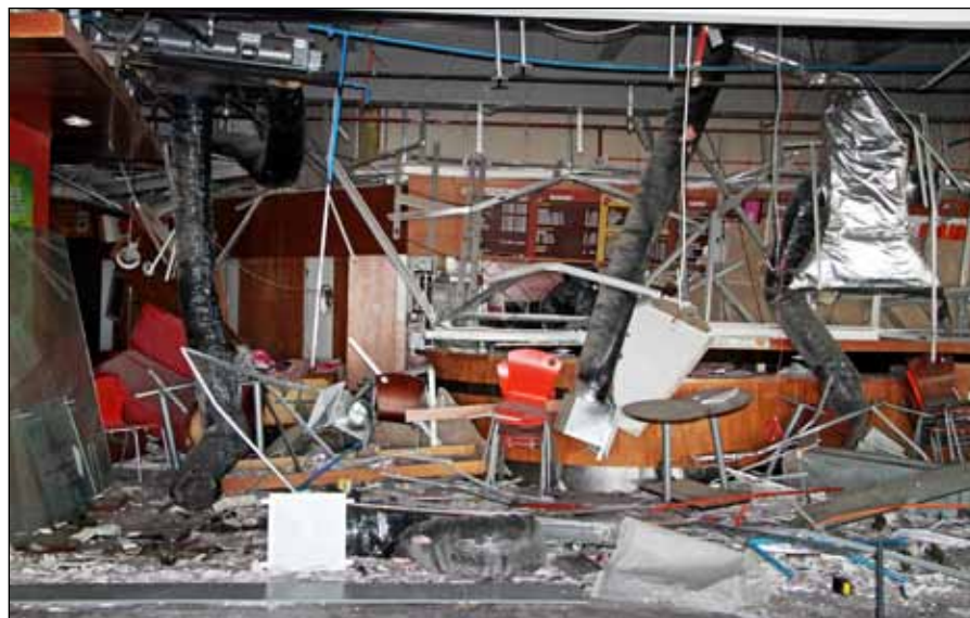
Figure 20. Nonstructural damage at the Santiago International Airport terminal (photo: E. Miranda).
