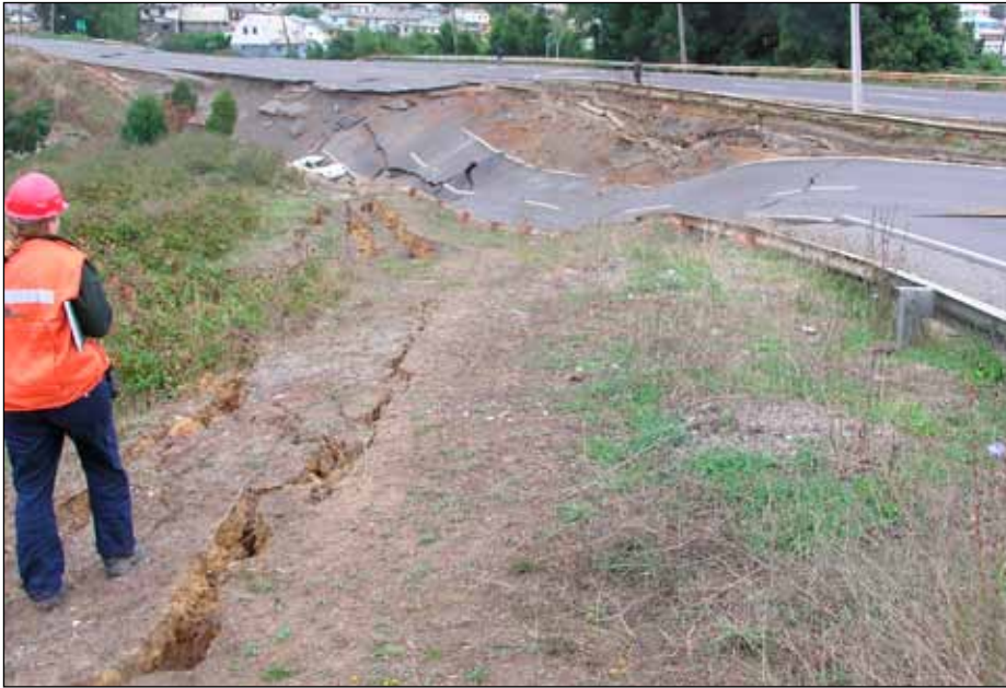
Figure 7. Slope failure on Route 160 in Lota (photo: GEER 2010).
