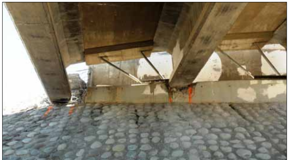
Figure 24. Lateral movement of the superstructure of Las Mercedes Bridge across Route 5 near Rancagua, due to absence of end diaphragms and transverse shear keys. Note extreme deformation of vertical seismic bars and damaged curtain walls (photo: Ministerio de Obras Públicas).
