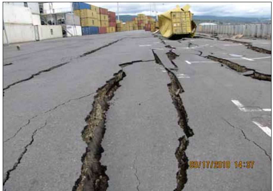
Figure 6. Liquefaction and lateral spreading-induced damage at the Port of Coronel (photo: GEER, 2010).
