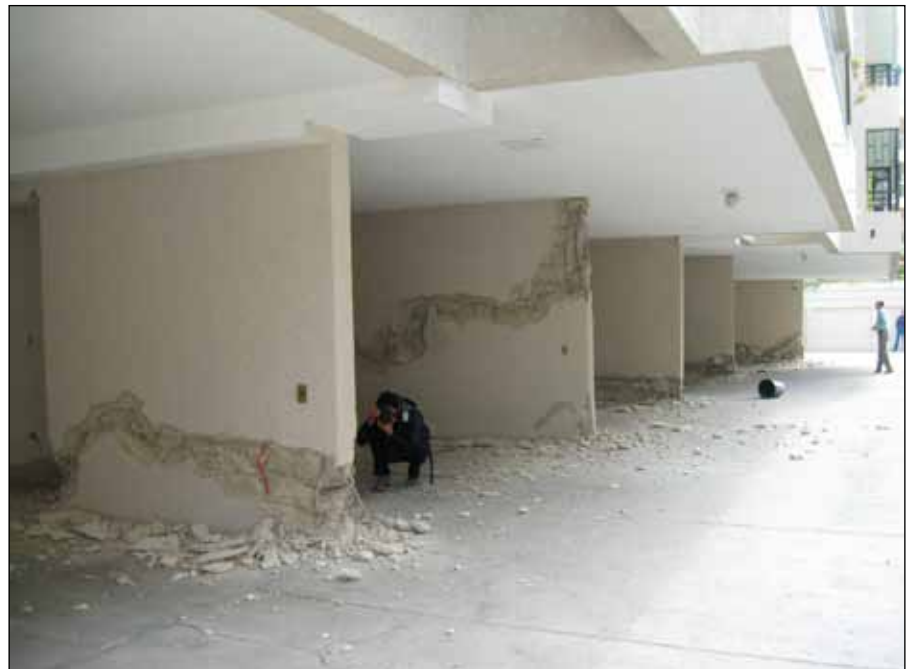
Figure 15. Wall damage, Viña del Mar (photo: P. Bonelli).
