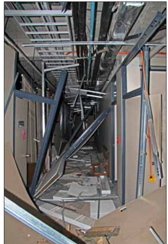
Figure 19. Nonstructural damage in the Talca Supreme Court building constructed in 2003 (photo: E. Miranda).
