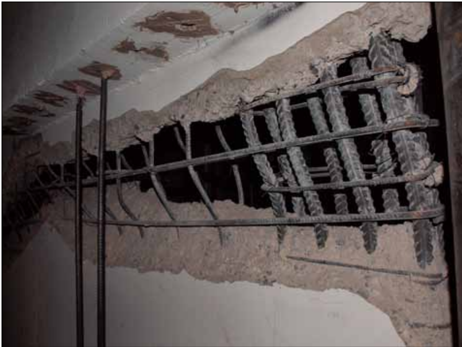
Figure 16. Wall damage, Santiago. Note the 90-degree bends on the transverse reinforcement (photo: J. Wallace).
