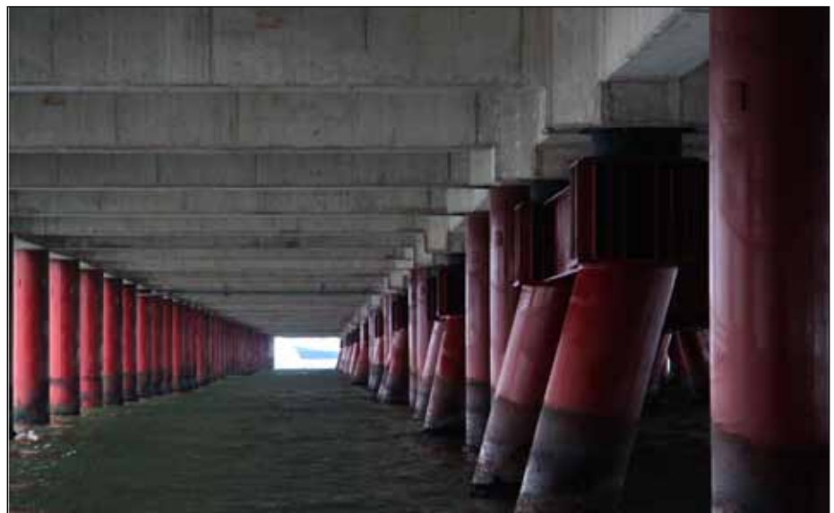
Figure 27. Base-isolated wharf at Coronel (photo: E. Miranda).
