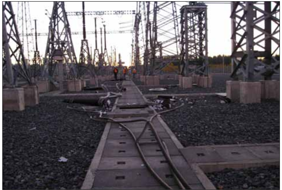
Figure 22. Damaged candlestick style live-tank circuit breakers (photo: TCLEE).
