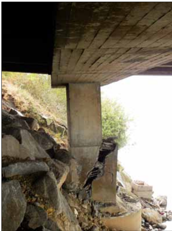
Figure 26. Shear failure in a column in northern approach to Juan Pablo II Bridge across Bio-Bio River, Concepción, due to lateral spreading and the propping action of the superstructure at the top of the column (photo: J. Arias).
