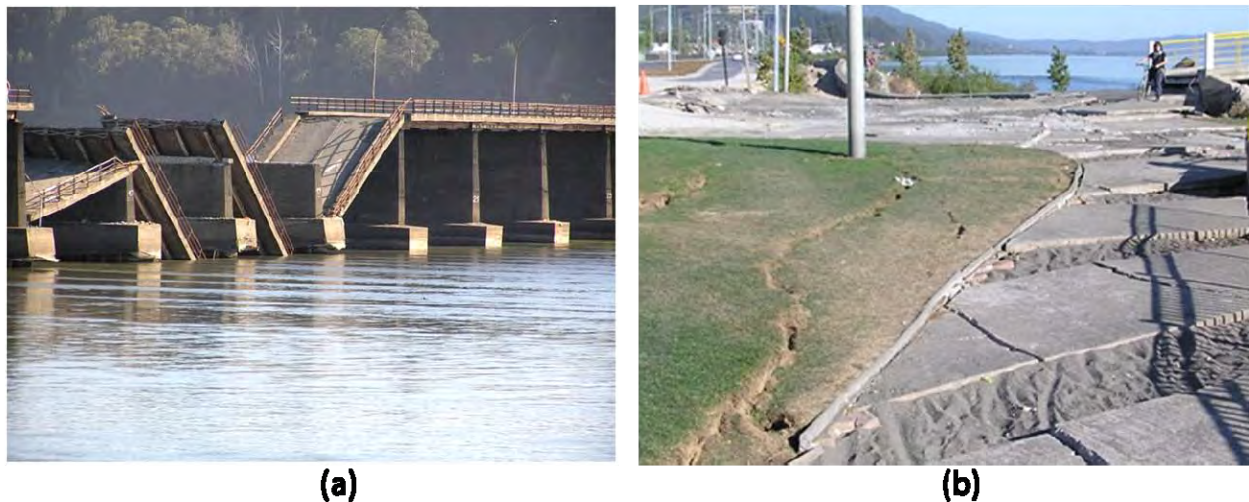
Figure 9.24. Puente Bio-Bio: (a) Collapsed slabs (S36.836789° W73.062203° on 3/15/2010), (b) Evidence of lateral spreading near East bridge approach (S36.837311° -73.061831°; 1753 hrs on 3/15/2010).
