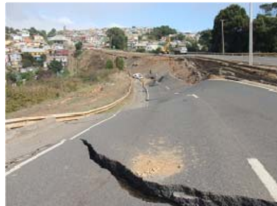
Photo 17 Big slide of road embankment in Lota Norte
