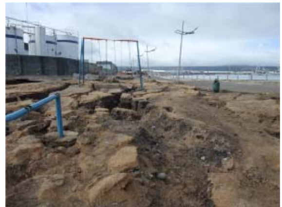
Photo 19 Lateral flow of soil adjacent to the pier
