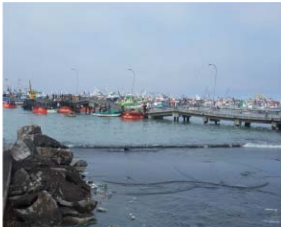
Photo 18 Damaged pier in Coronel
