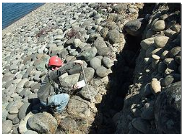
Photo 10 Downward slope movement in upstream face
