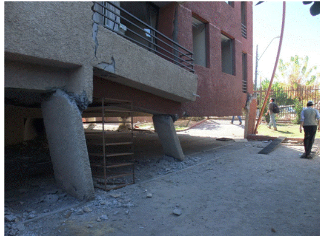
Photo 28 Collapsed building at Maipú in Santiago
