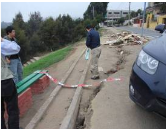
Photo 13 Minor slope failure at San Antonio
