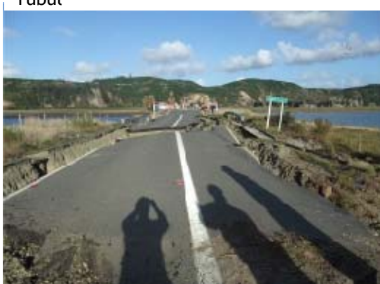
Photo 16 Collapsed approach embankment of Raqui II bridge
