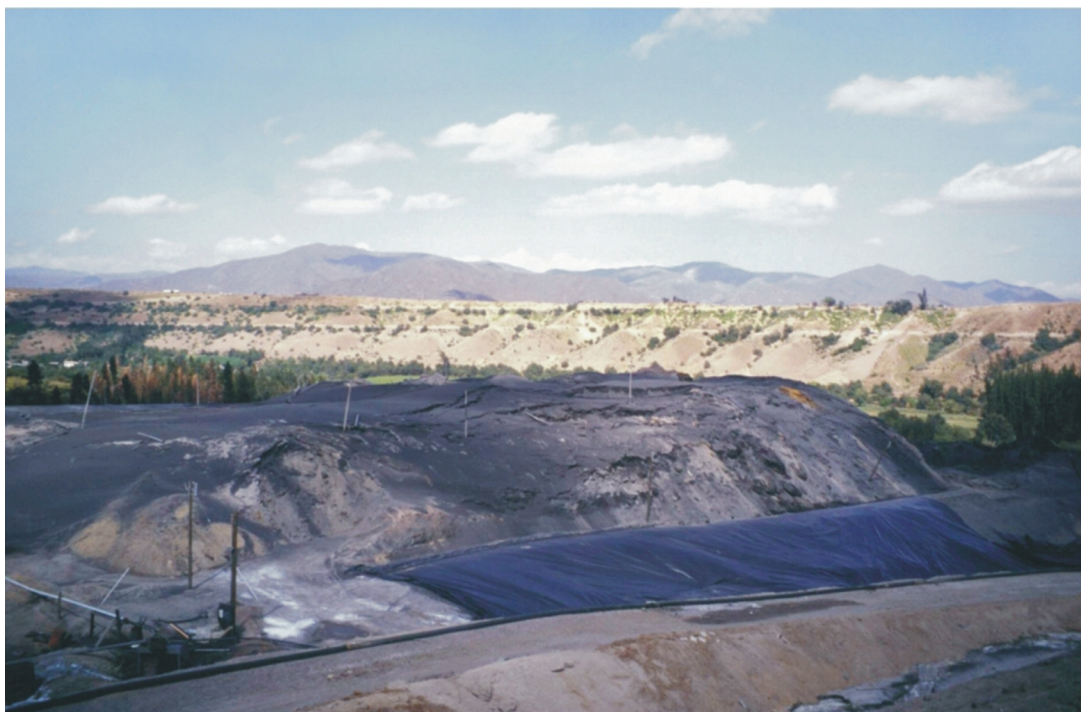
Fig. 7. Antiguo sand tailings dam at La Cocinera Plant, where slides and deformations were caused by the earthquake of 14 October 1997.
