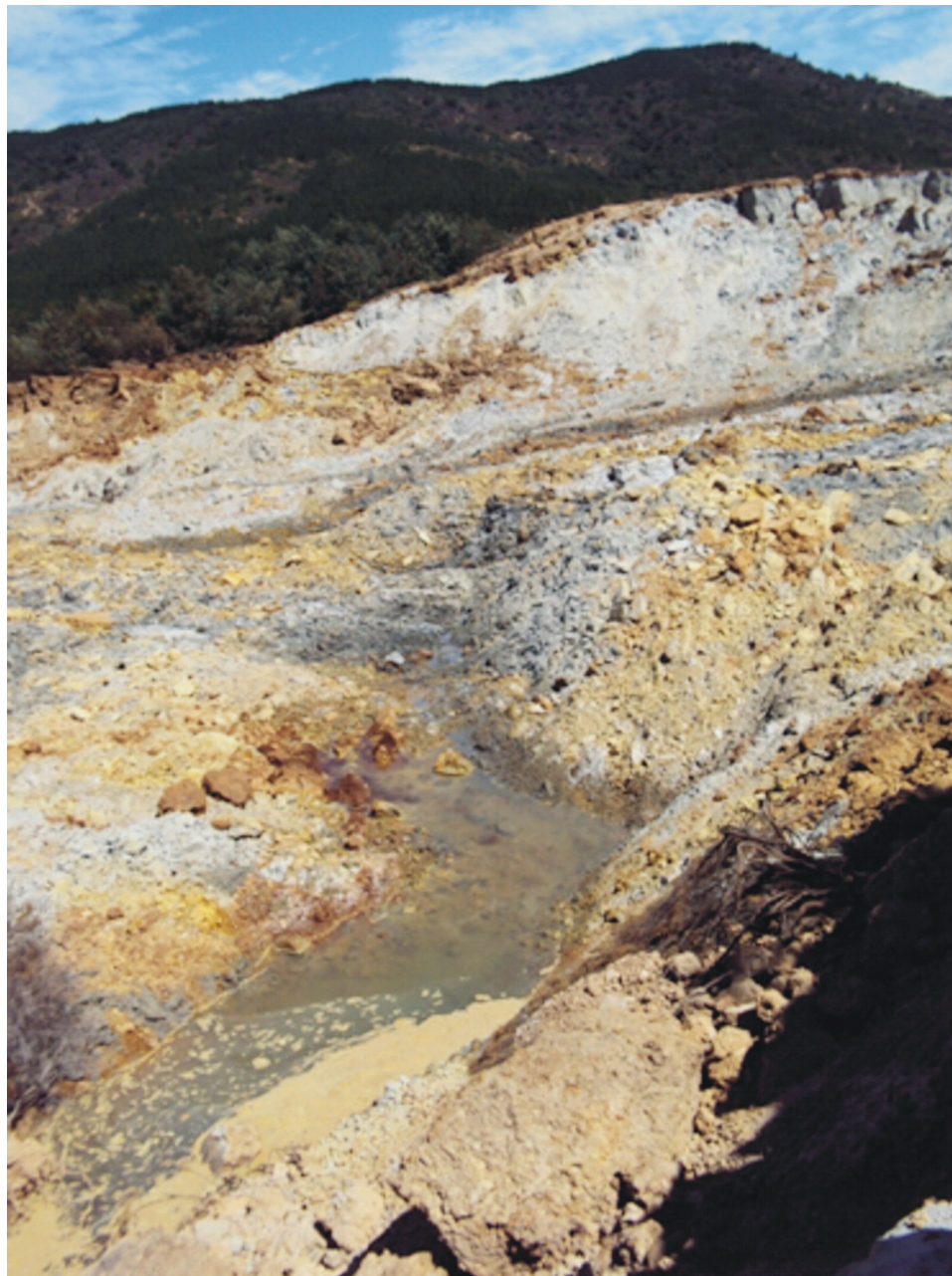
Fig. 9. Groundwater flow through the retaining dyke that collapsed at Las Palmas Dam.
