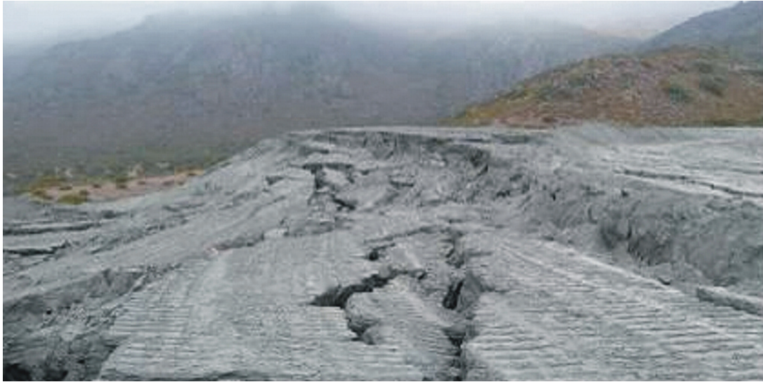
Fig. 5. Upstream slope deformations of retaining dyke caused by settling of underlying slimes.
