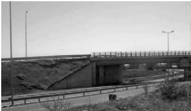
Figure 27. Surficial sloughing on a Route 5 overpass bridge approach embankment north of Chillán, with the abutment showing no evidence of damage.
