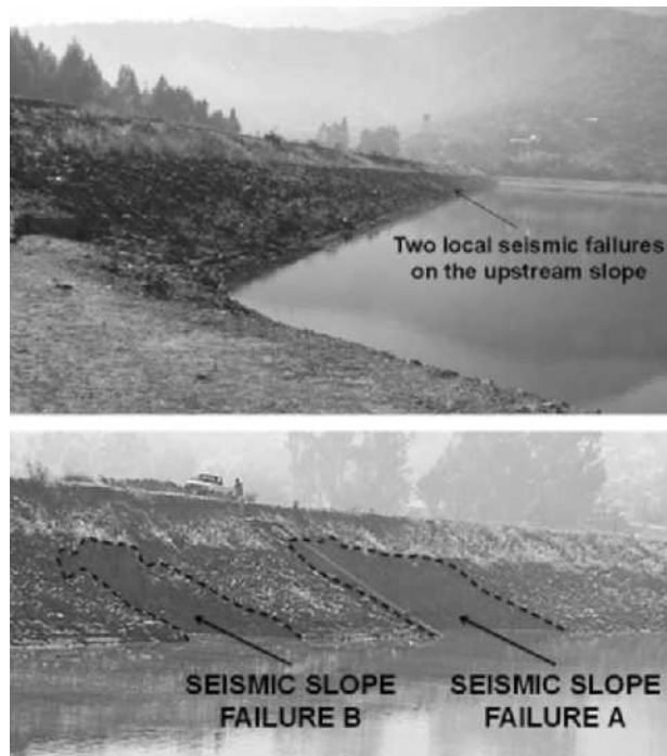
Figure 15. Seismic slope failures occurred in Lliu-Lliu Dam.
