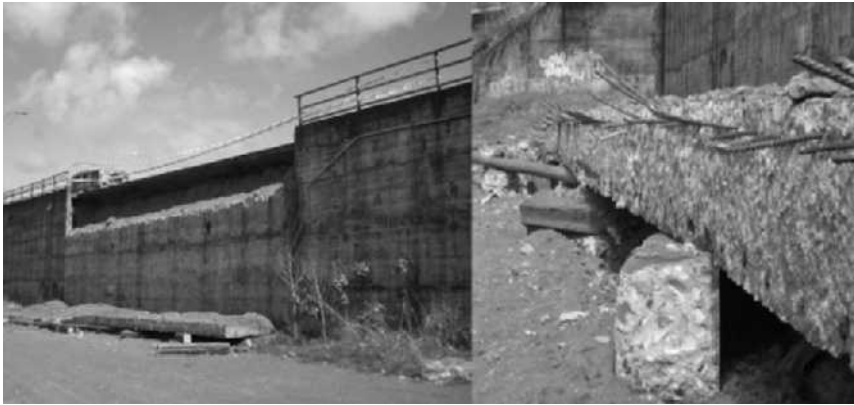
Figure 28. Failed reinforced concrete retaining structure in San Pedro. Failure occurred along a concrete “cold joint” and showed complete corrosion of the reinforcements (right photo).
