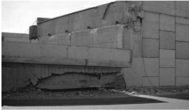
Figure 24. Intersection of Américo Vespucio Norte and Independencia, Santiago. The Reinforced Earth™ abutment performed well despite bridge collapse.
