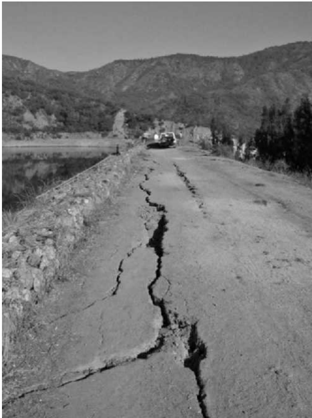
Figure 16. Open cracks observed along the crest of Lliu-Lliu Dam.
