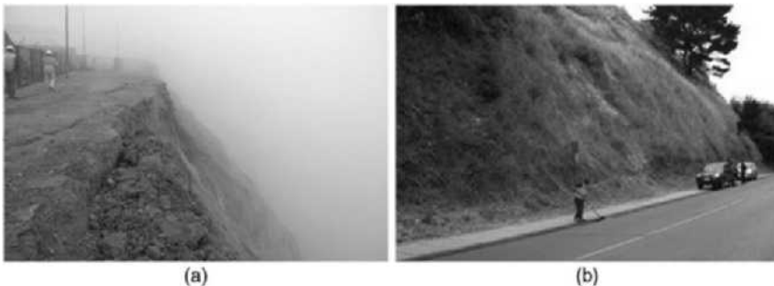
Figure 23. Steep slopes without evidence of major seismic displacements. (a) Near Barahona tailings dam. (b) City of Constitución.
