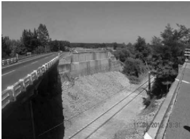
Figure 25. Reinforced Earth™ bridge abutments at a collapsed rail crossing on Route 5, north of Parral.
