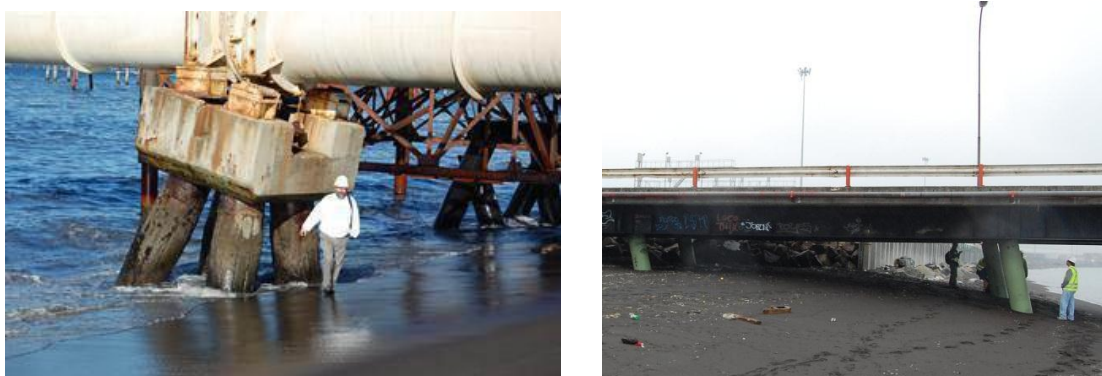
Fig. 20.- Damages observed in private infrastructure and Port of Coronel
