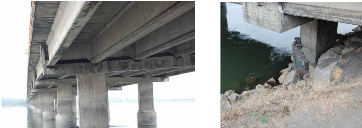
Fig. 17.- Settlement caused by liquefaction, and failure due to lateral spreading. Juan Pablo II Bridge affected by 2010 Chile Earthquake
