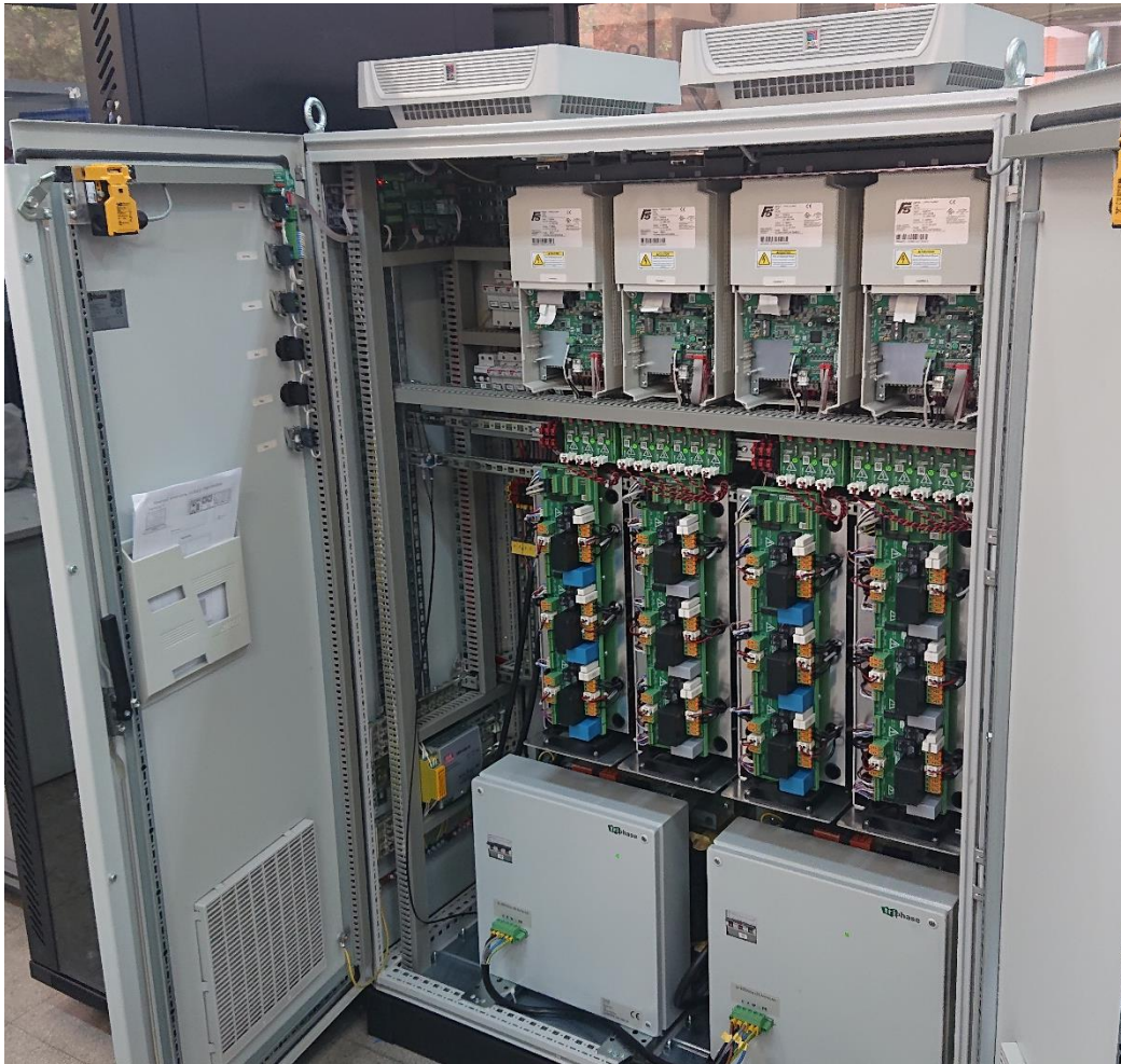
Inside a triphase unit
