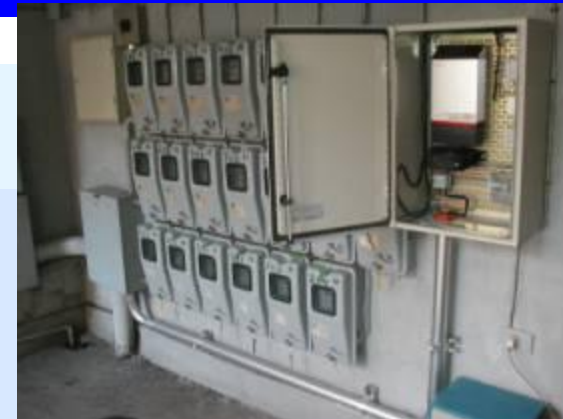
Ascom Repeater in Meter Room
