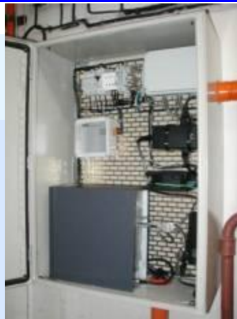
DS2 Repeater in Meter Room
