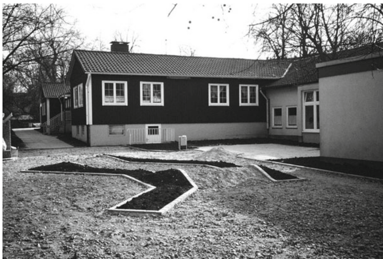
Fig. 5.7 Contaminated land overbuilt and sealed to interrupt the direct contact soil-human; photograph taken during the construction process in Oulu, Finland
