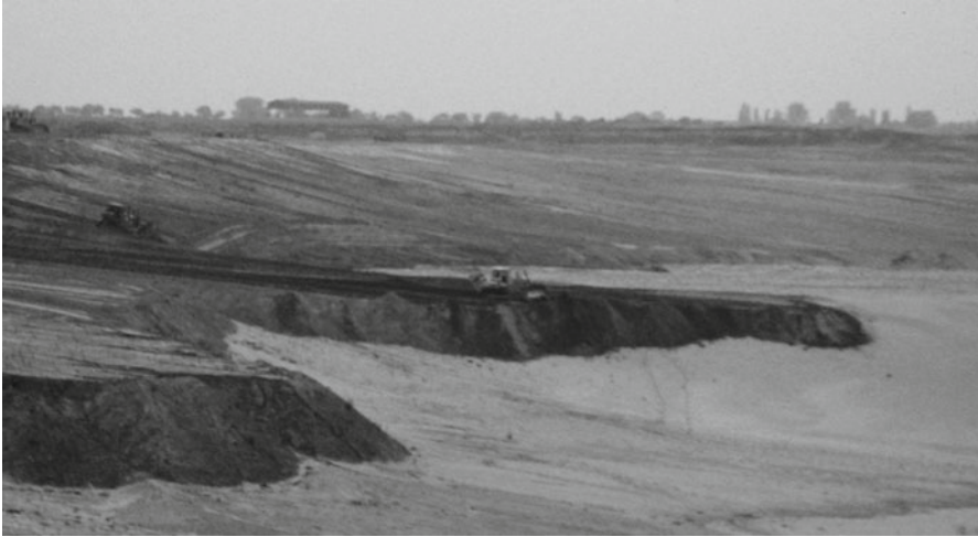
Fig. 3.9 Operation to design the shoreline of an artificial mining lake by means of vibrating rollers near Cottbus, Germany
