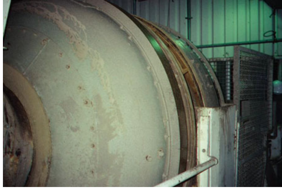
Fig. 6.7 Attrition equipment in a soil washing plant
