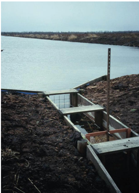
Fig. 3.41 Water basin for final collection of the overflowing water originating from plenty of polders
