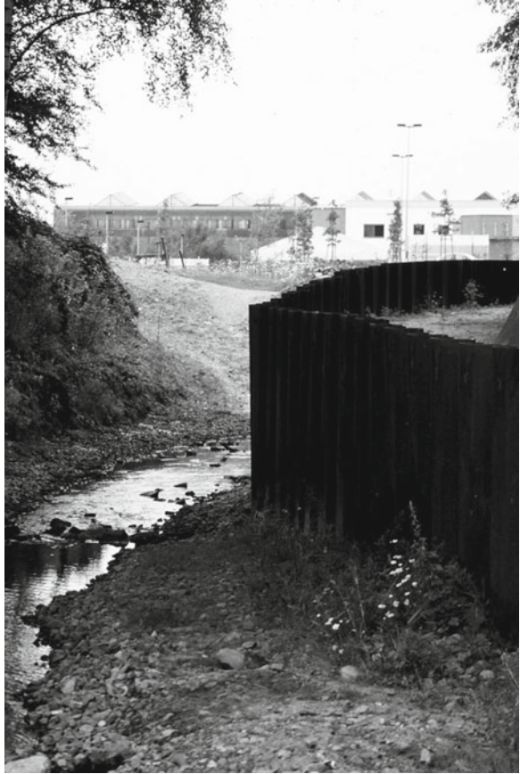
Fig. 5.8 Sheet pile wall of steel to protect a stream against erosion of contaminated soil
