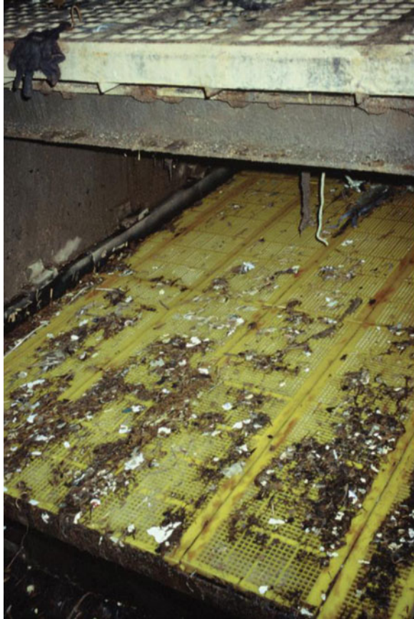
Fig. 6.8 Sieve cascade in a soil washing plant
