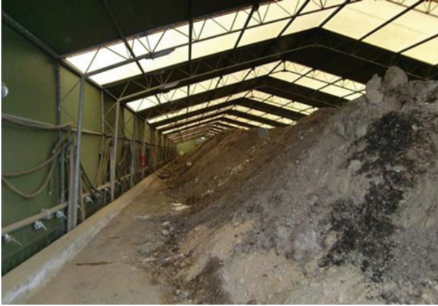
Fig. 6.17 Roofed regeneration pit (With kind permission of DHC company, Freiberg, Germany)
