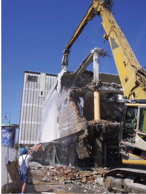
Fig. 4.15 Hydraulic excavator demolishing an industrial building; an employee tries to minimize dust development using a water hose (With kind permission of IGfAU company, Melle, Germany)
