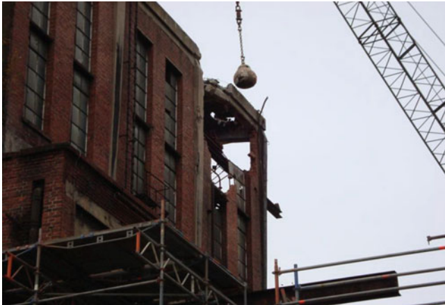
Fig. 4.16 Ball crane demolishing an industrial building (With kind permission of IGfAU company, Melle, Germany)
