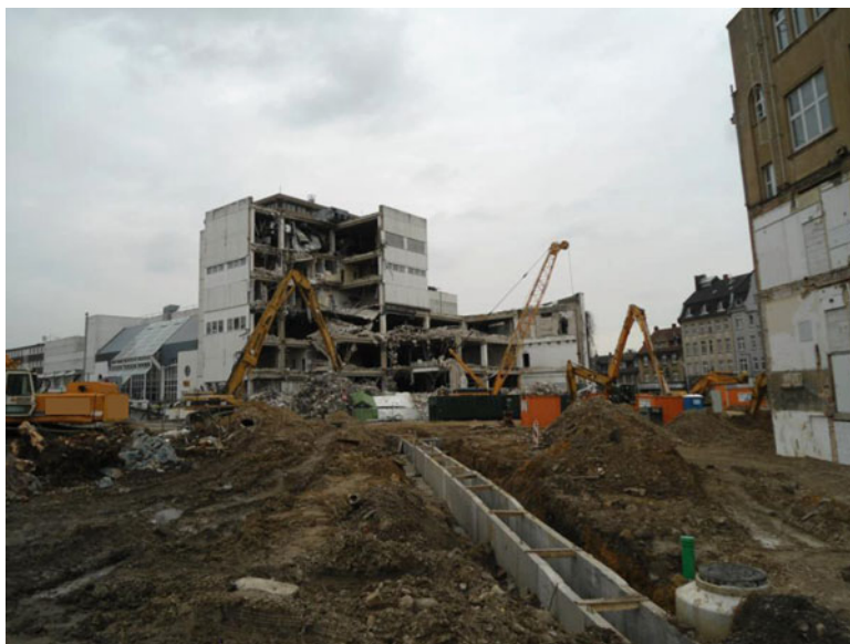
Fig. 4.22 Demolition of a contaminated building (in the background ) simultaneously to the construction of a side barrier (arranged in the foreground ) (With kind permission of IGfAU company, Melle, Germany)
