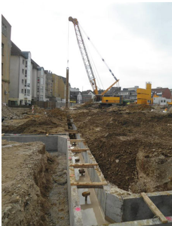
Fig. 5.11 Hydrofraise installing a side barrier to minimize pollutant migration into an adjacent residential area (With kind permission of IGfAU company, Melle, Germany)
