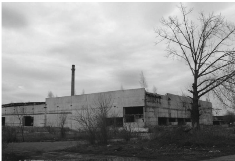
Fig. 4.23 Damaged contaminated industrial building in Pernik, Bulgaria, before demolition occurs
