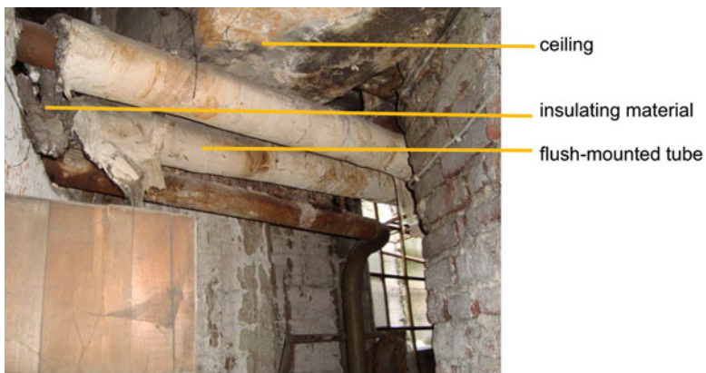
Fig. 4.19 Flush-mounted insulating material which may be contaminated (With kind permission of IGfAU company, Melle, Germany)
