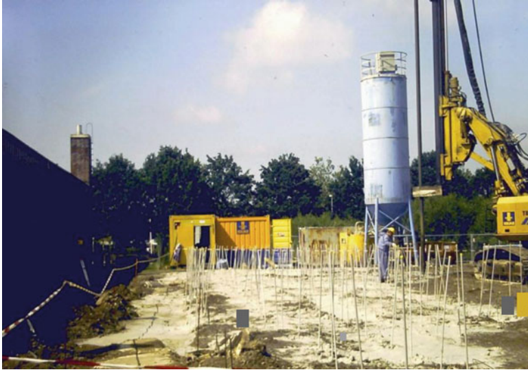
Fig. 5.14 Horizontal sealing by tube injection; the slurry (stored in the container) is pumped into the white tubes which are arranged close together (With kind permission of Wessling company, Altenberge, Germany)
