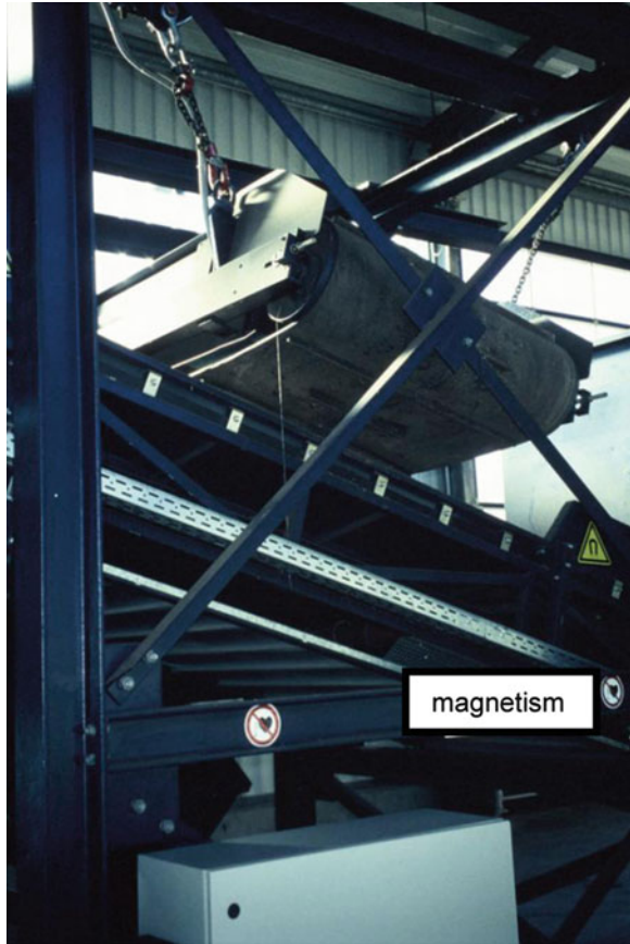
Fig. 6.5 Magnetic overhead belt separator to detach ferrous metals
