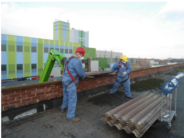
Fig. 4.24 Workers with full protective clothing who dismantle cement asbestos panels (With kind permission of IGFAU company, Melle, Germany)
