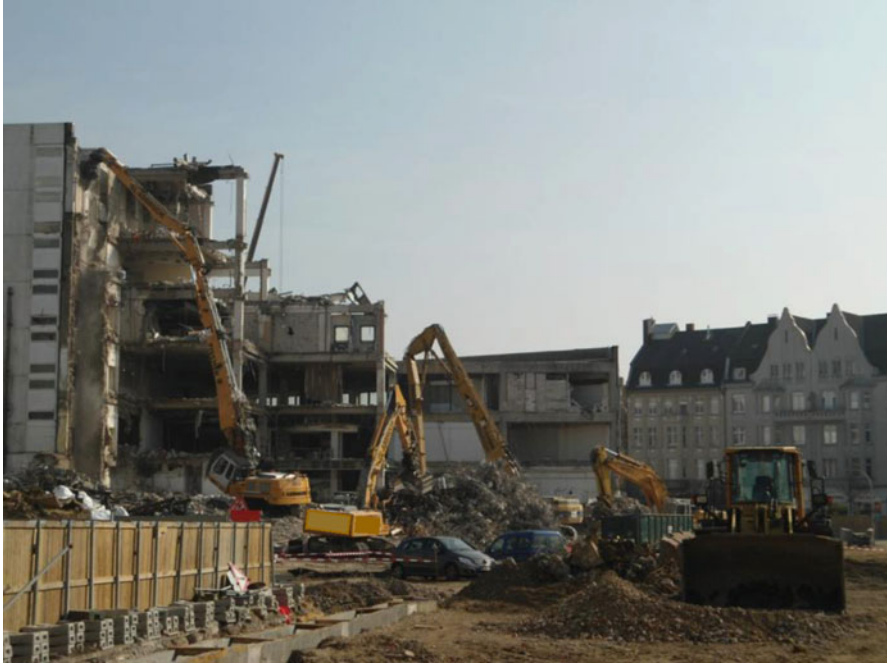
Fig. 4.17 Demolishing excavator with shear attachment ( left ), hoe ram and crawler excavator ( centre ) as well as bulldozer ( right ) in full operation (With kind permission of IGfAU company, Melle, Germany)
